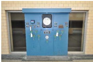
Existing 1958 Filter Control Console
