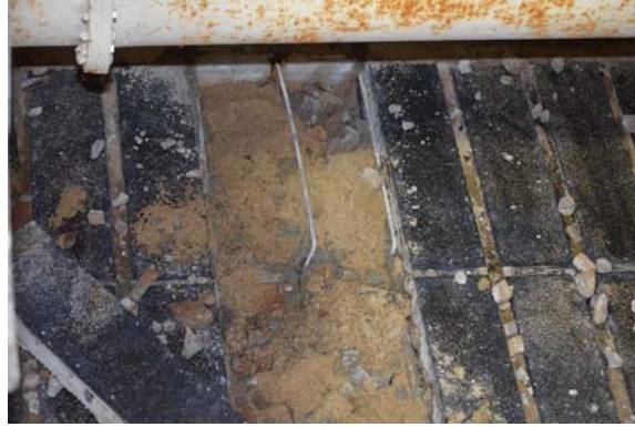
Infiltrated Media in Failed 1930 Filter
