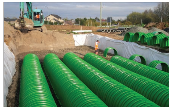
Example of underground basin installation
